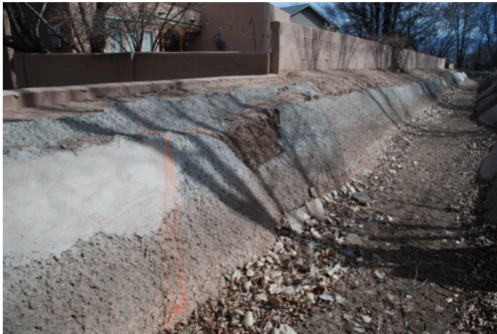
Example of sidewall failure, previous patch. Area inside orange line Replaced entirely.
